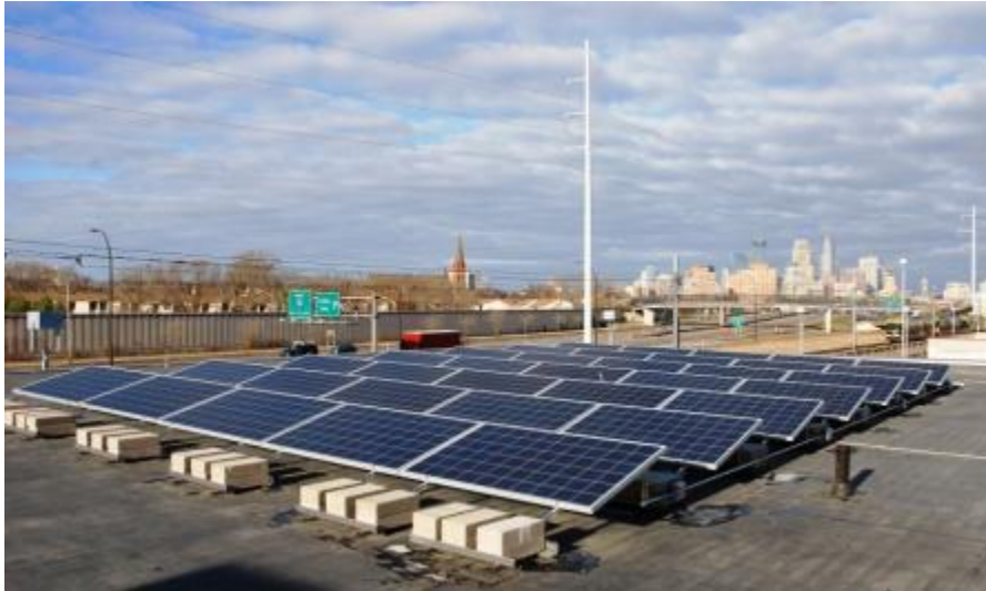
Figure 2 Solar Array at Metro Transit Light Rail Facility
