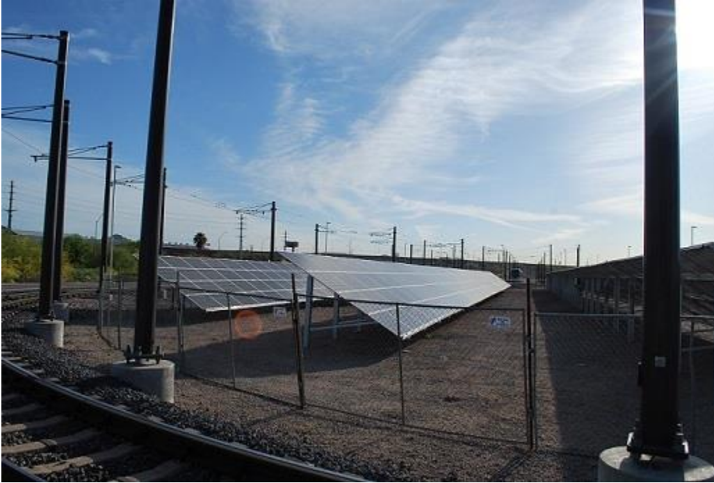
Figure 3 Ground-Mounted Solar Array at Valley Metro
