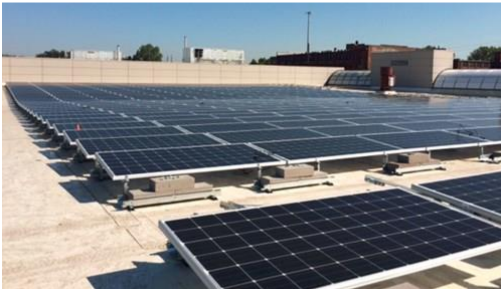
Figure 1 IndyGo Solar Array
